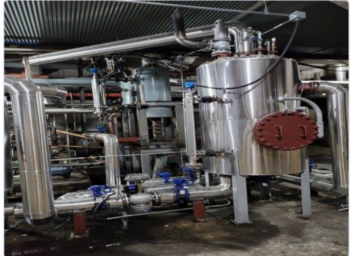
A group separator and its pipework
